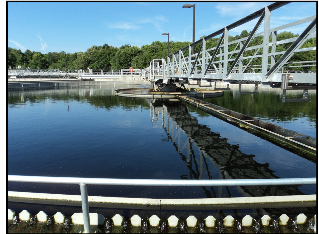
Effluent Clarifier at the Triangle Wastewater Treatment Plant
