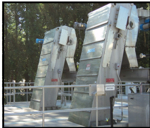
Fine Bar Screens at TWWTP
